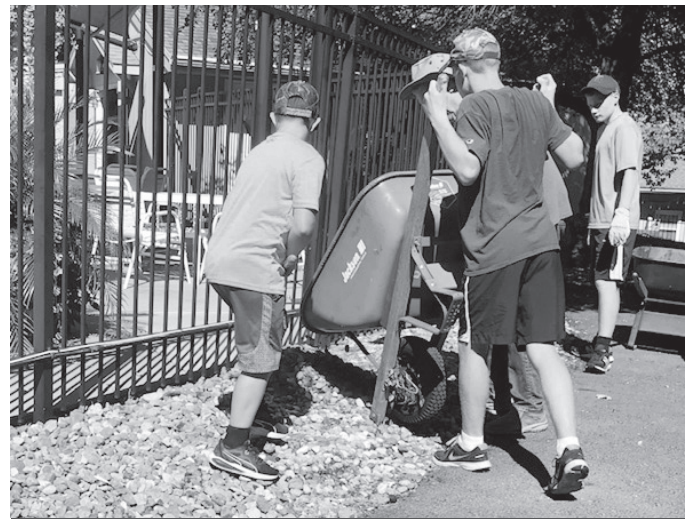
Northwood Trails kids Joel, Daniel, Nathan and Caleb Wuertz worked hard this summer to help improve the grounds by mulching along the pond dam and hauling wheel barrows of rock to spread along the pool fence.
